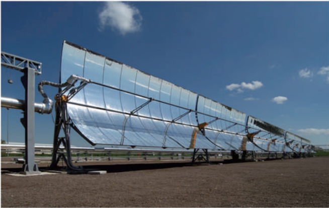
槽式集热系统 Parabolic Heat Collecting System
