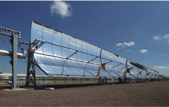
槽式集热系统 Parabolic Heat Collecting System
